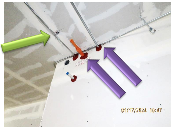
One electrical pipe was properly supported, while the other electrical (and orange pipe) was not.
