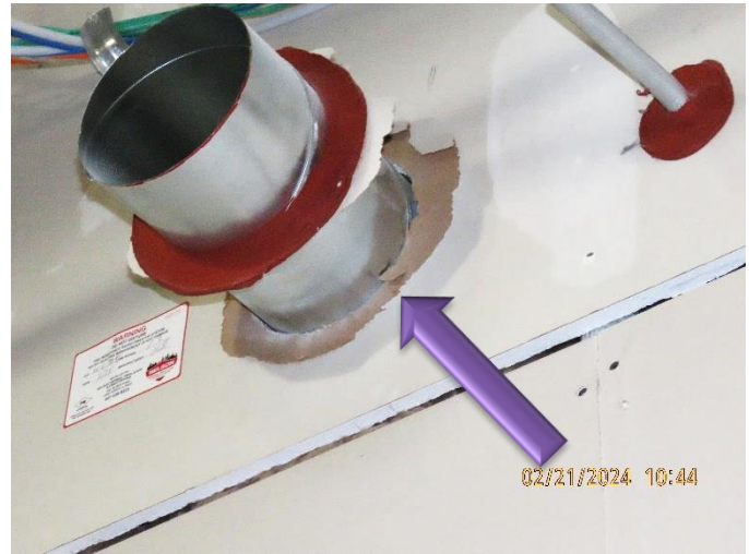
The round mechanical duct has been moved during the installation of the next component after the fire stopping was installed.
